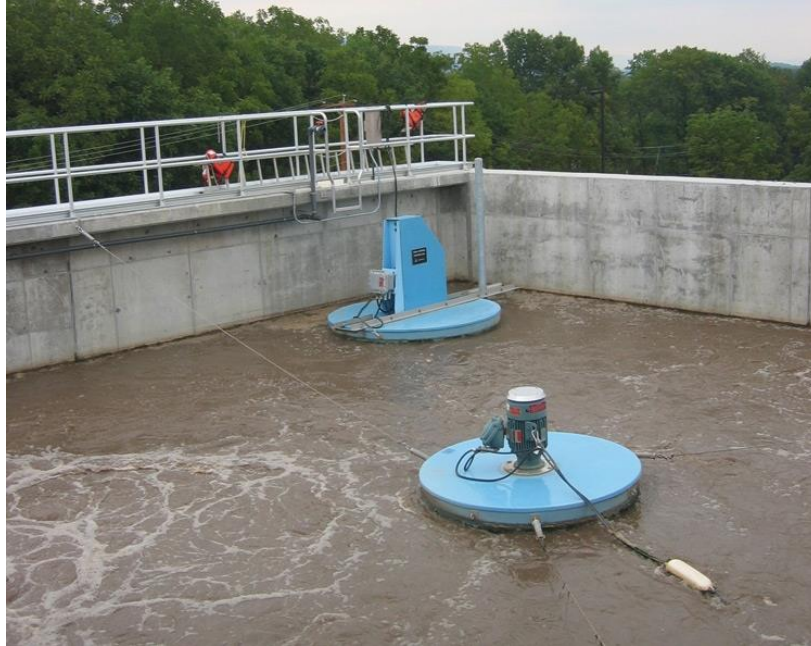
Figure 4.21: SBR Tank w/Surface Mixer/Aerator and Decant Device (Credit: Aqua-Aerobic Systems, Inc.)
